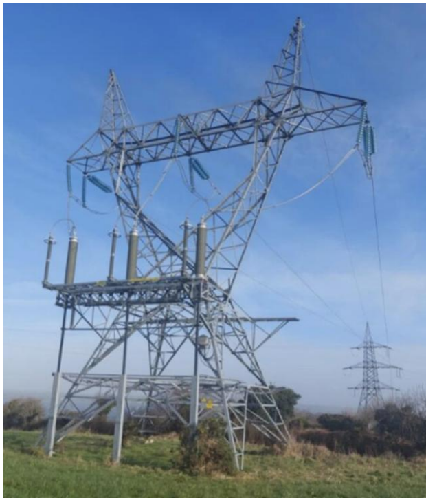
Figure 2.6: Line Cable Interface Mast (LCIM)
